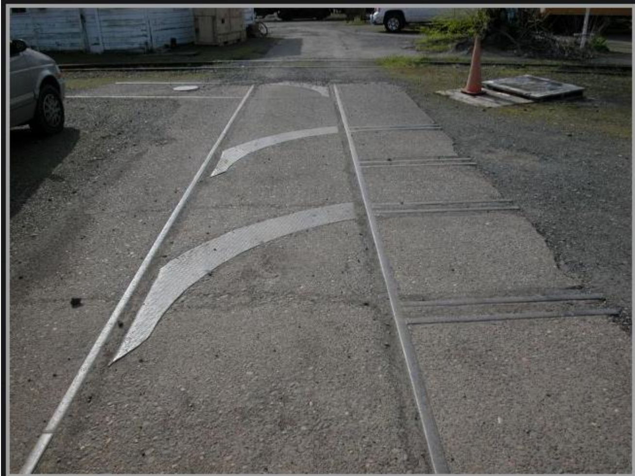
These were guides for helping wheelsets make 90 degree turns when moving between roundhouse and backshop. Photo by Terry Thompson.
